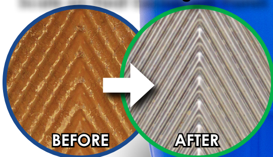
Scale on Heat Exchanger Plates
