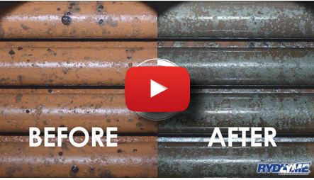
Watch as RYDLYME Descaler safely and efficiently removes scale from boiler tubes!
