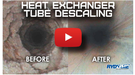
Watch as RYDLYME Descaler dissolves scale build up from this heat exchanger tube!
