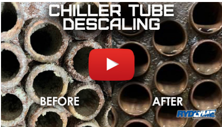
Watch as RYDLYME Biodegradable Industrial Descaler dissolves scale build up from this chiller!
