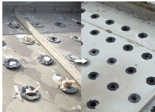
Cooling tower (hot deck) at an institutional facility
